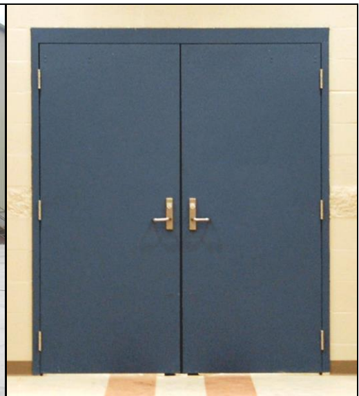
Hollow Metal Doors and Hardware
